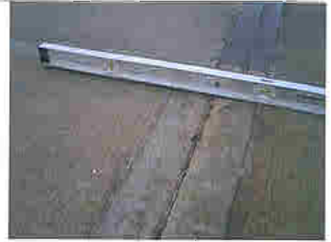
1 inch wide joint at the end of the tied arch span closed up as a result of the bridge deck system moving outward.
