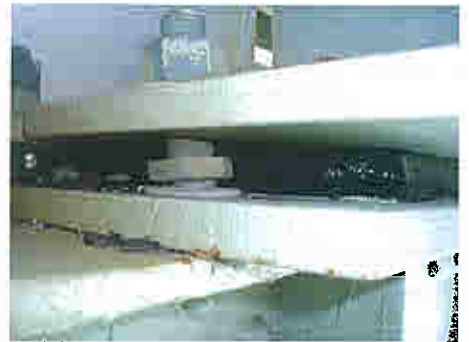
Stringer bearing and its anchor bolt being pushed towards the end of the tied arch causing extreme deformation of the elastomeric bearings and shearing of the bearing anchor bolts.
